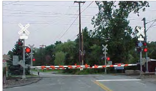
Four Quadrant Gates at the School Street crossing on the Northeast Corridor High Speed Rail Line in Mystic, CT. (Volpe Center photo)
